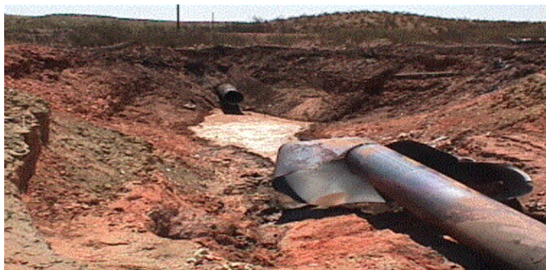
Figure 3. Recent USA Pipeline Failures (36) in Bellingham, 1999 (top) and New Mexico, 2000 (bottom) (Images courtesy of the National Transportation Safety Board, USA)
