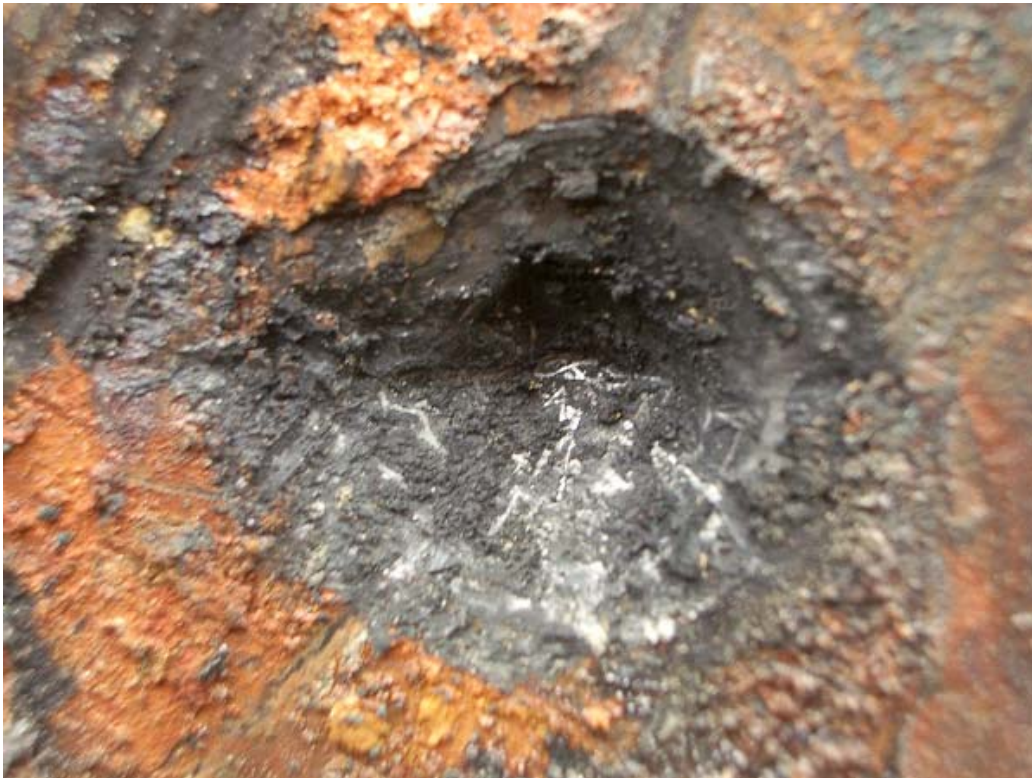
Figure 4 Microbially Induced Corrosion
