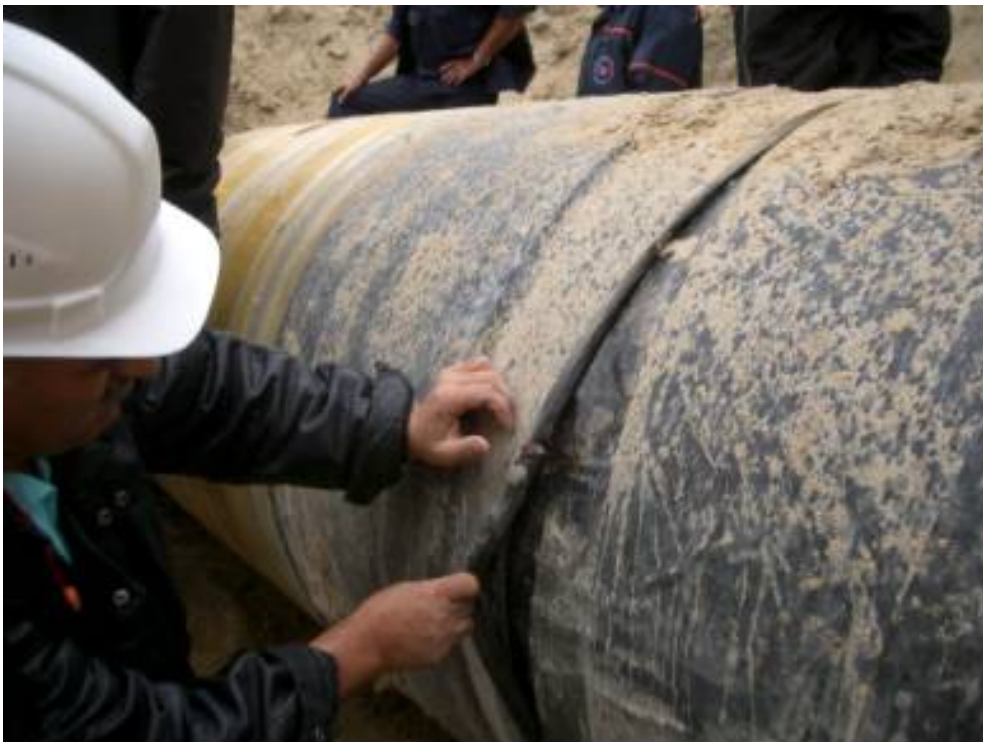
Figure 8 Poorly adhered tape refurbishment coating
