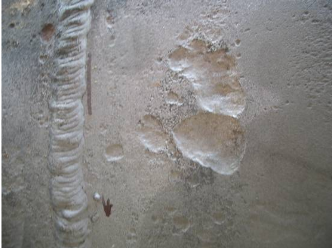
Figure 2 Example of external corrosion
