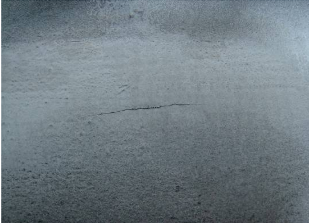
Figure 4 Example of a manufacturing defect
